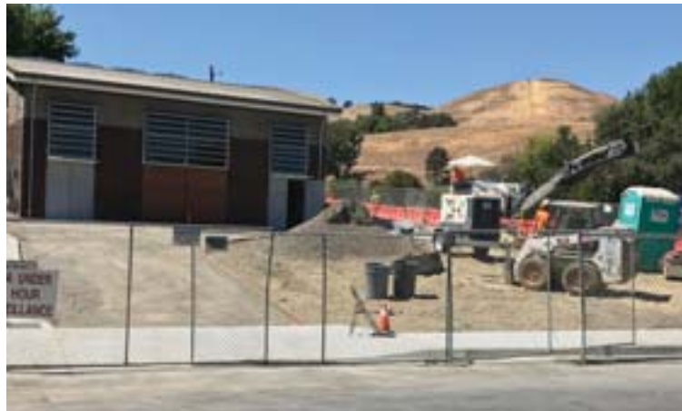
EBMUD's new Diablo Vista pumping plant set to be operational by early 2018. Photo Pippa Fisher
